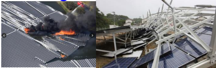
Collapse due to strong wind, electric shock, fire
