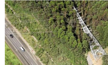
Collapse of power lines
